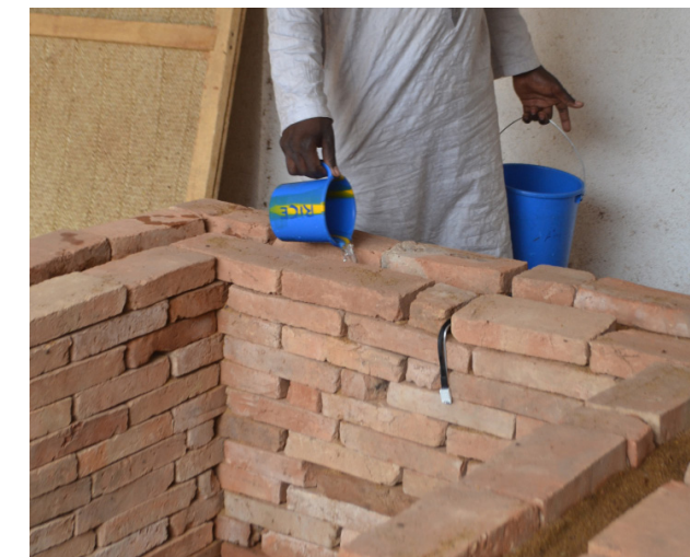
Adding water to an evaporative cooling chamber in Bamako, Mali.
